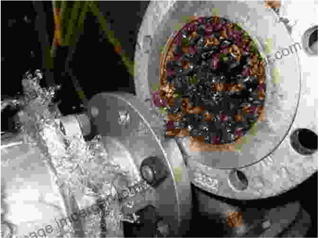
Clogged Water Intake
